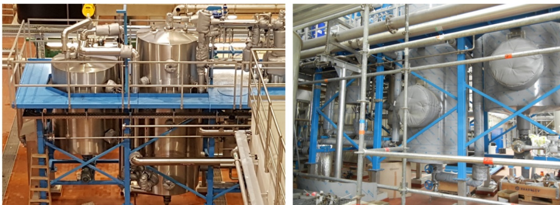
Figure 21 Pictures of the thermal pressure hydrolysis units (Haarslev process).
